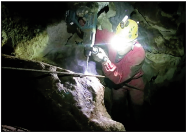
Photo 2: Chris putting in some bolts in the Olympian Cavern, Wombeyan Caves, 5-9-2017. Photo: Peter Bauer.
